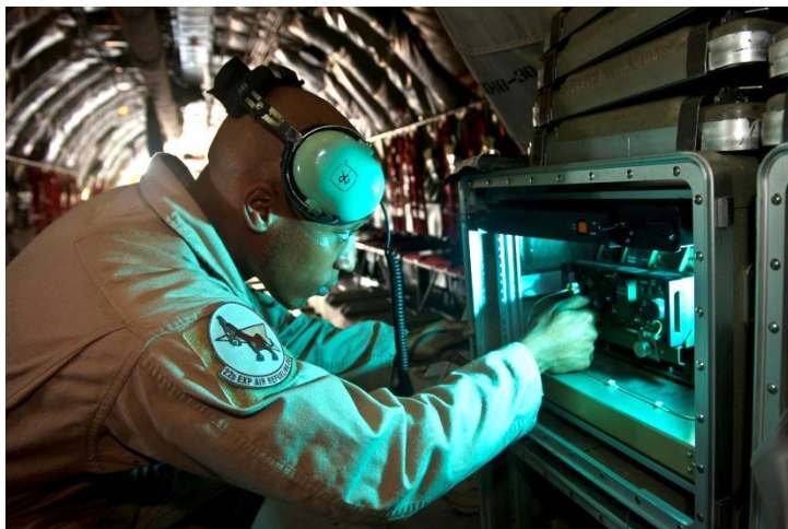
Airman 1st Class Nate Hammond adjusts the frequency of a Roll-On Beyond Line of Sight Enhancement, or ROBE, data link system at the Transit Center at Manas, Kyrgyzstan. A ROBE connects manpower assets on the ground to other ground or airborne units. (U.S. Air Force photo/Senior Airman Brett Clashman)
