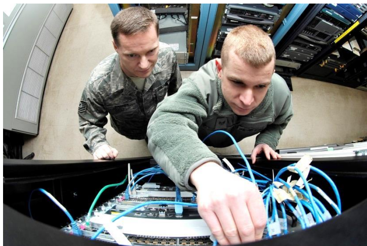
Air Force Tech Sgt. Kevin Garner and Air Force Senior Airman David Solnok, cyber transport technicians assigned to the 354 th Communications Squadron, hook cables in to the new Air Force Network router system at Eielson Air Force Base, AK. (U.S. Air Force photo by Staff Sgt. Christopher Boitz)
