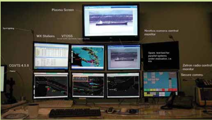
A Vessel Traffic Service workstation displays various means used to monitor maritime traffic including Coast Guard Vessel Traffic System, Automatic Identification System, radar and closed-circuit television. U.S. Coast Guard photo by Petty Officer Nathan Bradshaw.
